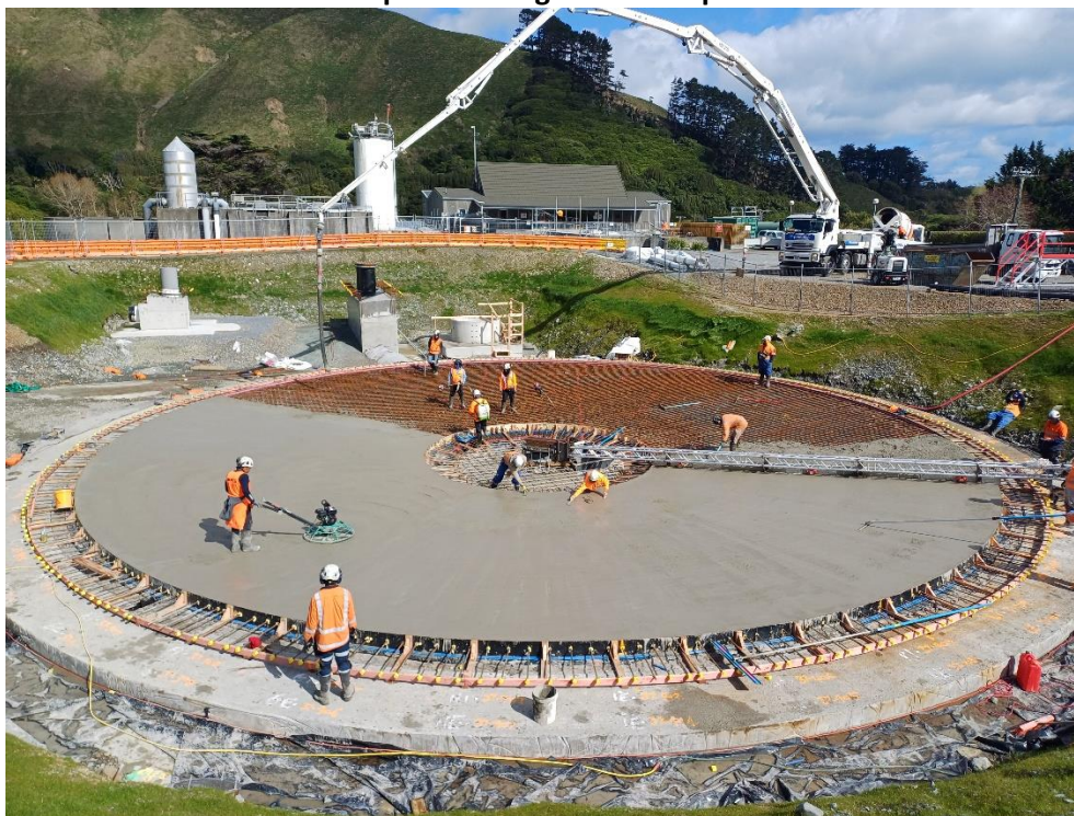
The screed follows the placement of concrete and allows for the finishing teams.
